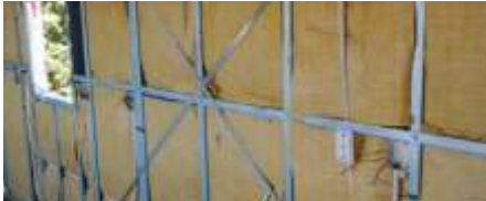
Cavity Bat Insulation
